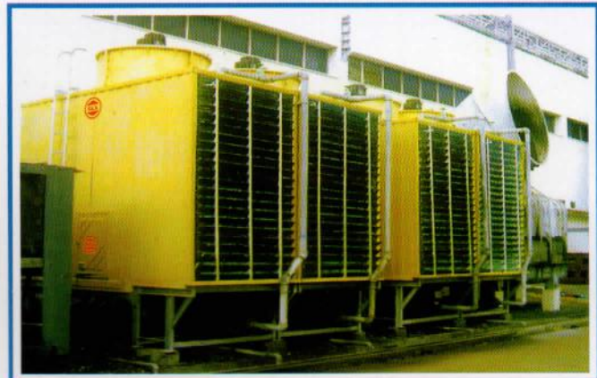
CLOSED CIRCUIT PACKAGED / FRP / Sony Dvice Technology (Thailand) Proj.
