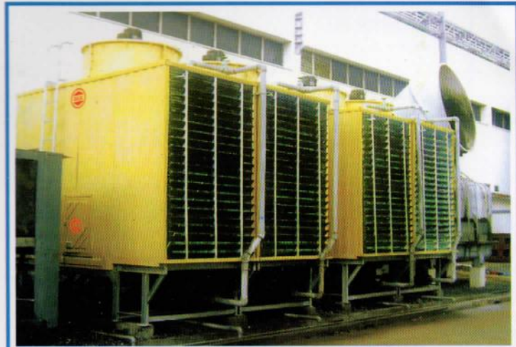
Sony Device Technology (Thailand) Project (BKC-C-125RT x 4 Cells)
