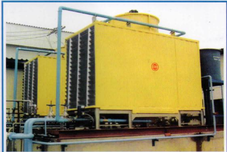
K.E.I. Engineering (Site I.C.P.) Project (BKC-C-100RT x 2 Sets)
